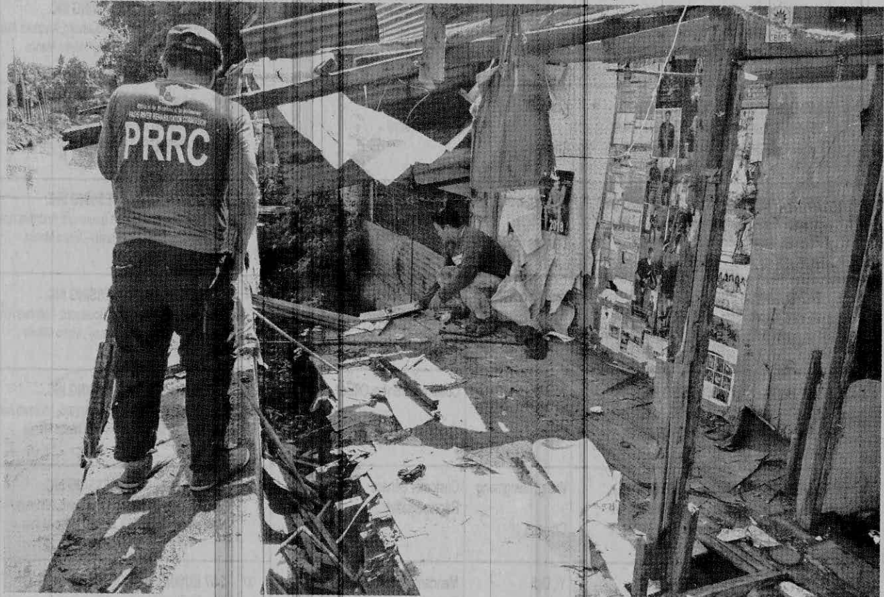
A MEMBER of the River Patrols dismantles the settlements and obstructions to begin the 145 meters of Ermitaño Creek linear park. PHOTO COURTESY OF PRRC
